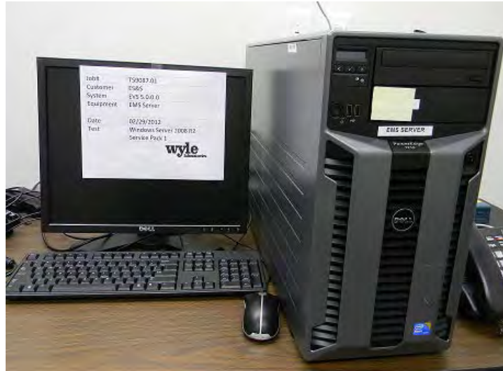
Photograph No. 6: EMS Server
