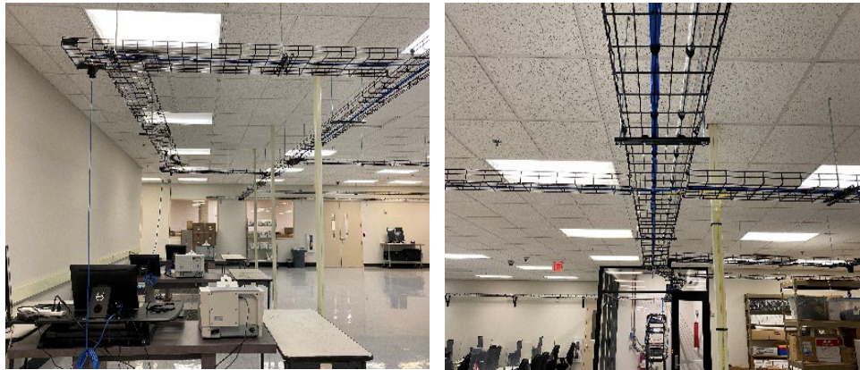
Tabulation Room – Secure Racking with Exposed Wiring
