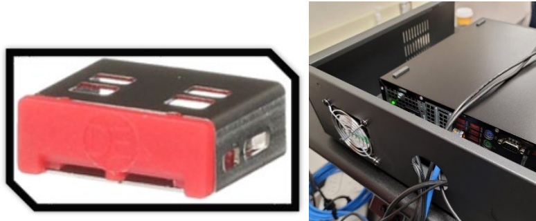
Tabulation Room: Customized Serialized Port Blockers (Left) and Security Canisters (Right)
