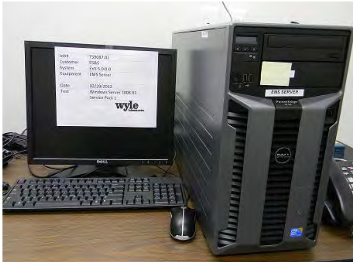
Photograph No. 6: EMS Server
