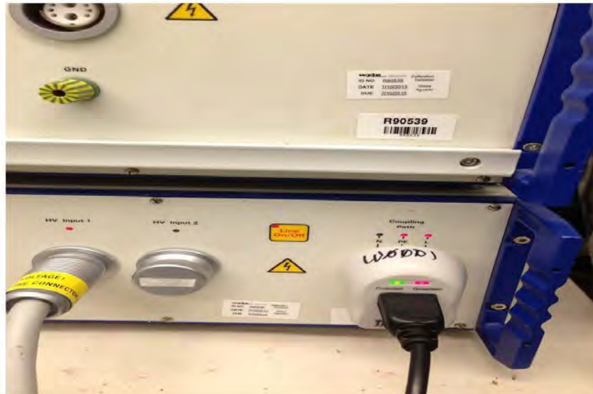
Photograph 12: ES&S FL EVS 4.5.0.0 Lightning Surge
