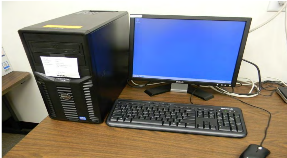
Photograph No. 7: EMS Server
