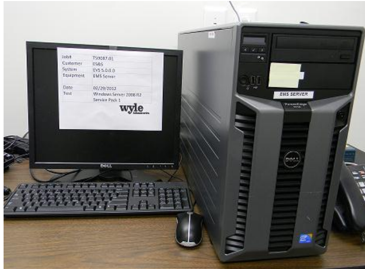
Photograph No. 6: EMS Server
