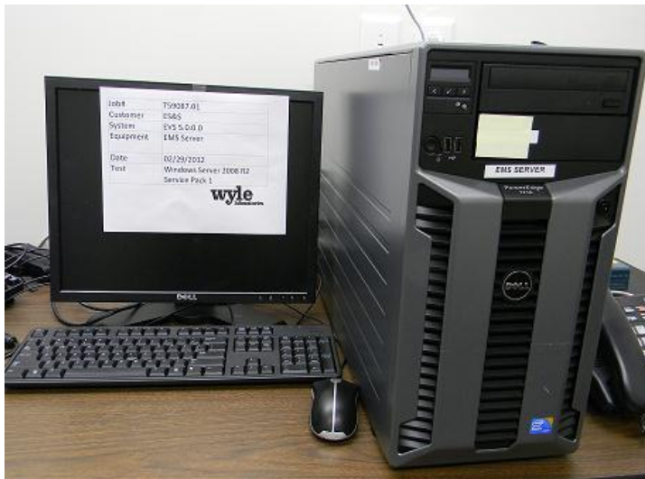
Photograph No. 10: EMS Server
