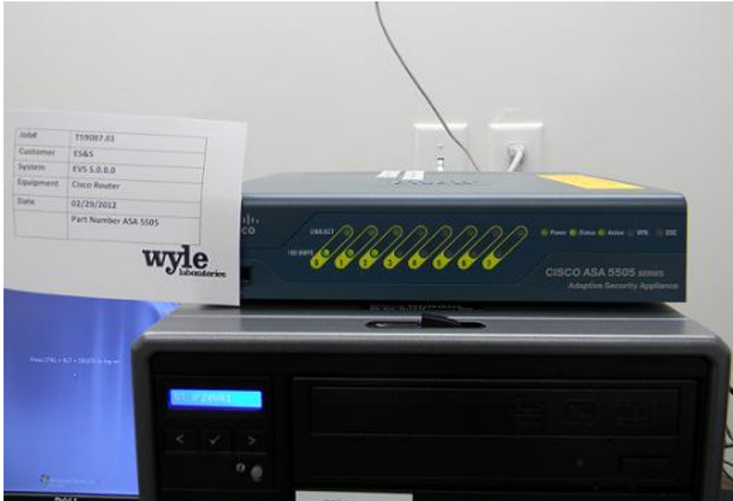
Photograph No. 8: Cisco Router Front View
