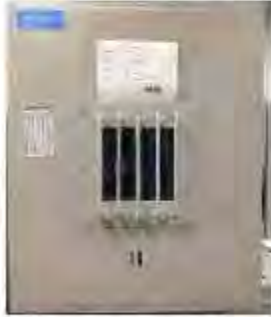
Photograph No. 34: 1S65 FL EV5 4.5/00 High Temperature
