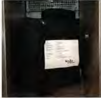
Photograph No. 33: 1S65 FL EV5 4.5/00 High Temperature
