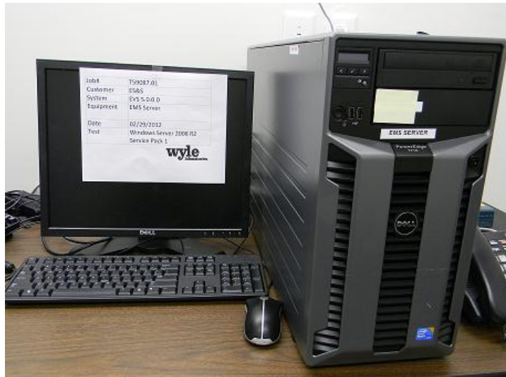
Photograph No. 6: EMS Server
